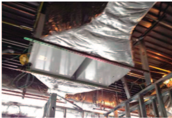
Two units were bundled to purify the air in this IVF lab in Chapel Hill, NC.
